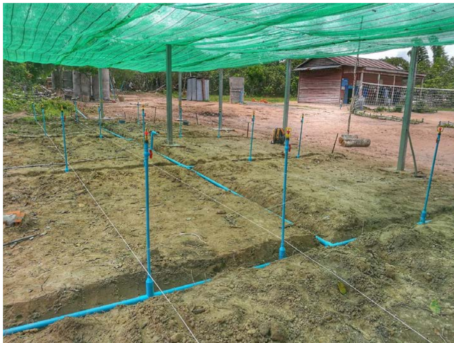
Water system and Tree nursery, under construction at Sangke Lak primary school.
