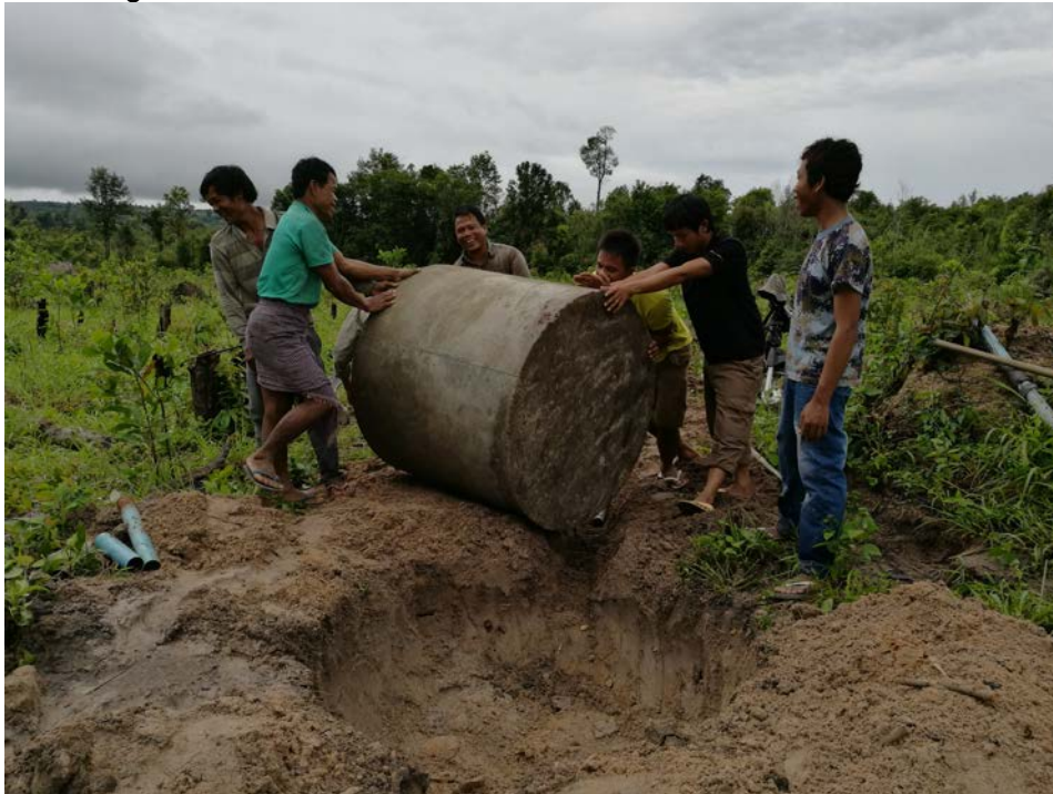
Setting up of the water system for Sangke Lak water system, November 2016.
